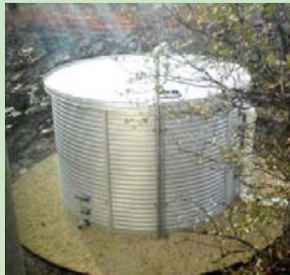
The rainwater harvesting system.
